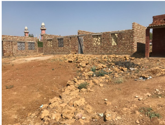
The first buildings of the new primary school. The roof is still missing.
