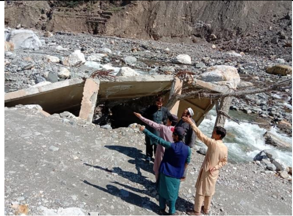
Road to the Dubair valley showing destruction
