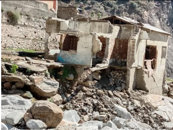
A house near a school is almost destroyed
