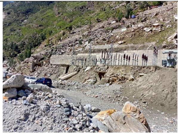
Flood damaged Electric Power Station in Dubair
